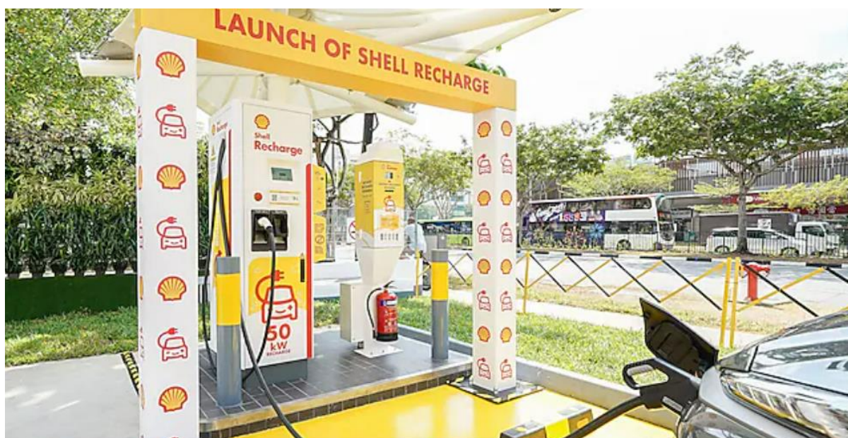
Shell launched Singapore's first electric vehicle charger at a service station, Shell Recharge, at Shell Sengkang. Shell Recharge will be available at nine other Shell stations by October 2019.
