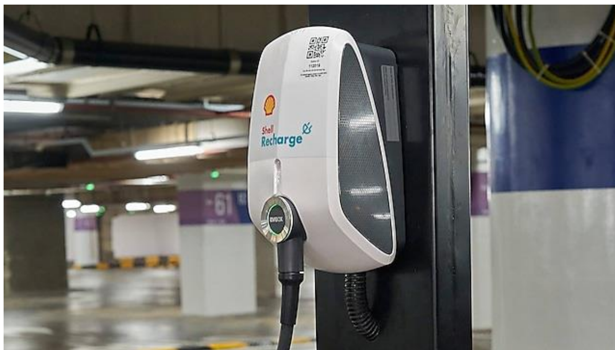
A Shell Recharge AC charger installed in a carpark
