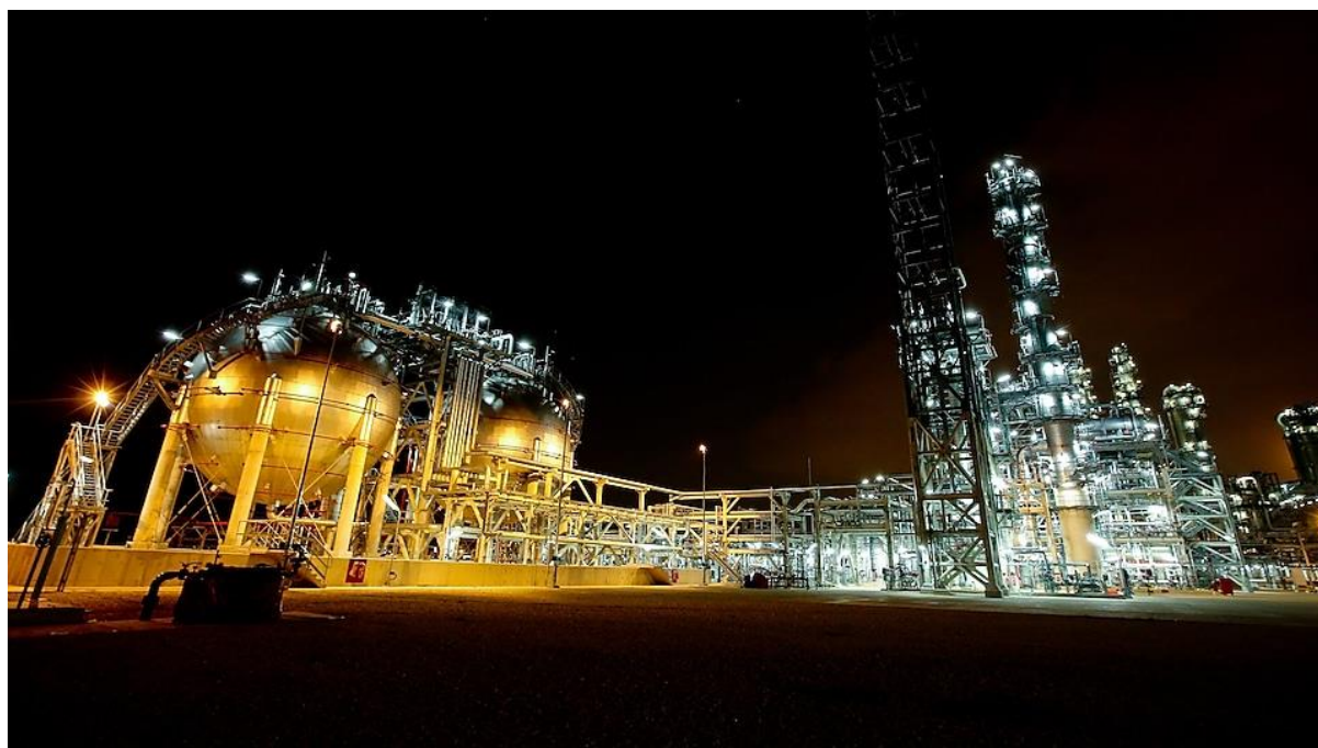
Shell's new purification unit on Jurong Island has the capacity to produce 140,000 tpa of HPEO.
